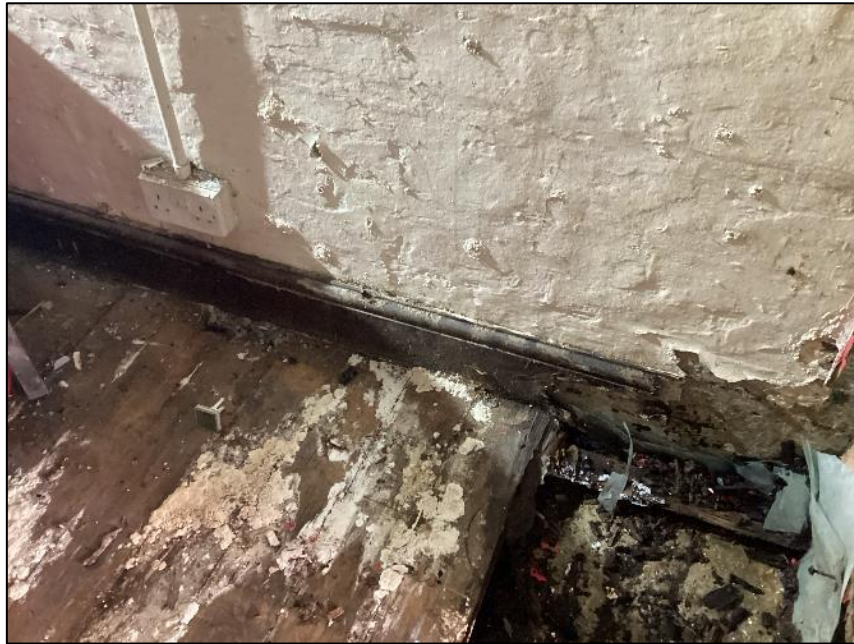
Plate 12. Rotten floor and skirting in the back function room
